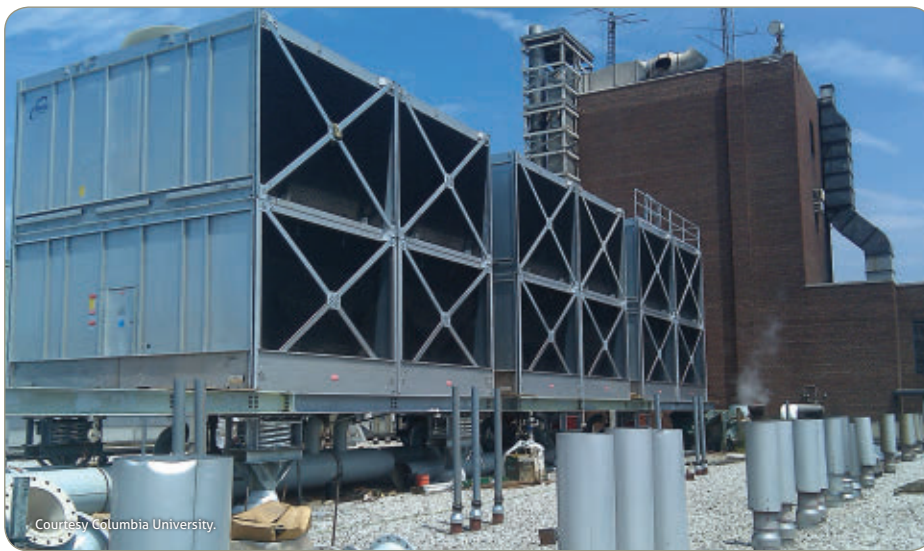
In 2011, new cooling towers were installed as part of Columbia’s Old Powerhouse chiller plant renewal.
