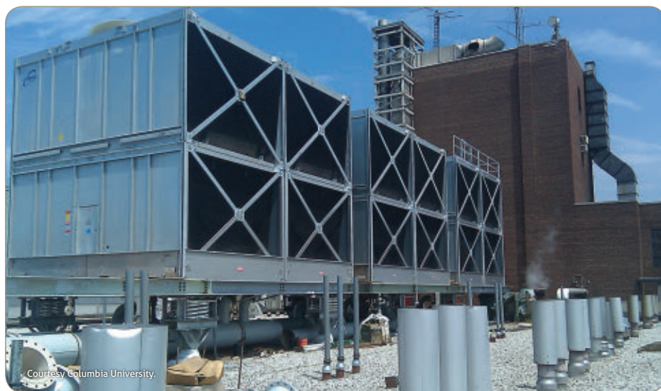
In 2011, new cooling towers were installed as part of Columbia’s Old Powerhouse chiller plant renewal.
